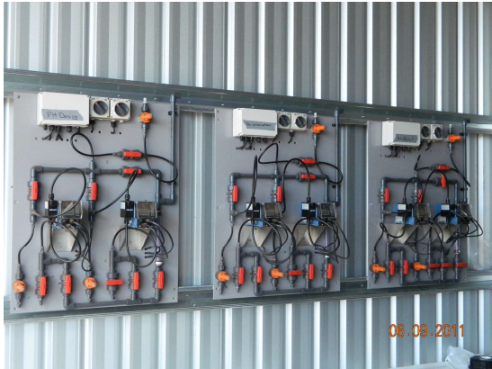
Image: Antiscalant, Sodium Hydroxide, and chlorination dosing panels.
