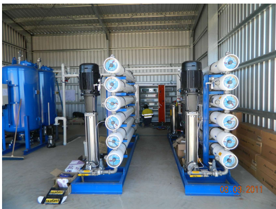
Image: Installed 2x 300KLD M83 RO racks, and PTI filters.
