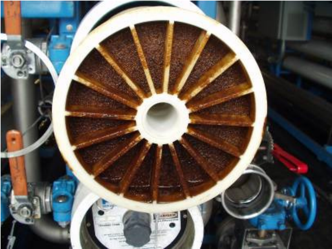
Picture 1 The RO elements with fouling on the membrane surface and on the feedwater inlet and out let sections of all of the elements.
