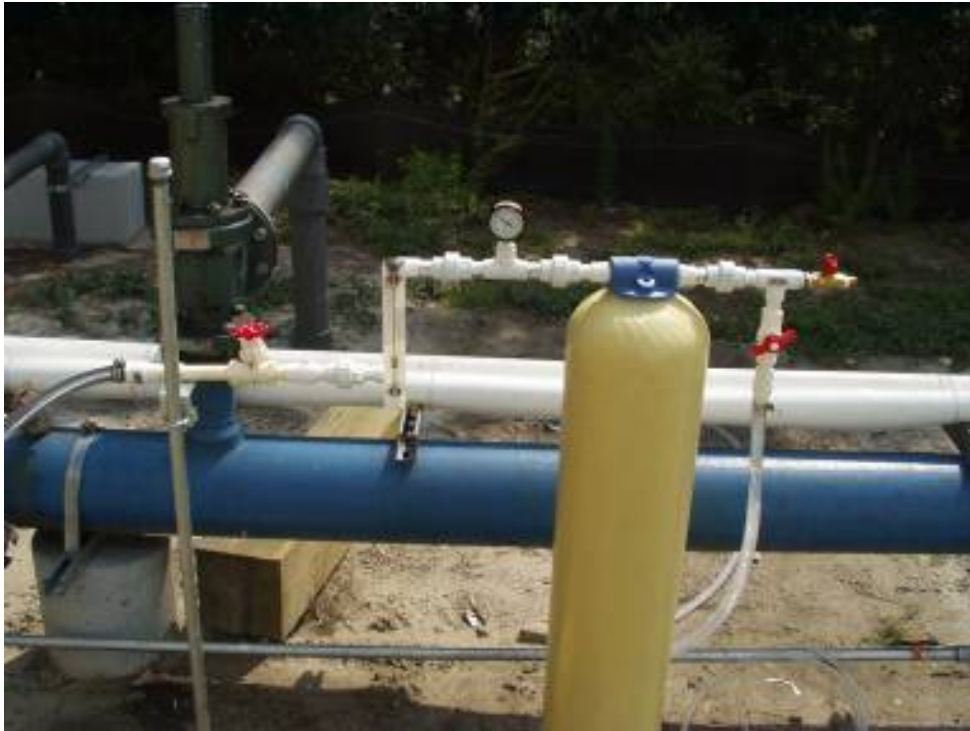
Picture 3: Filter test unit
