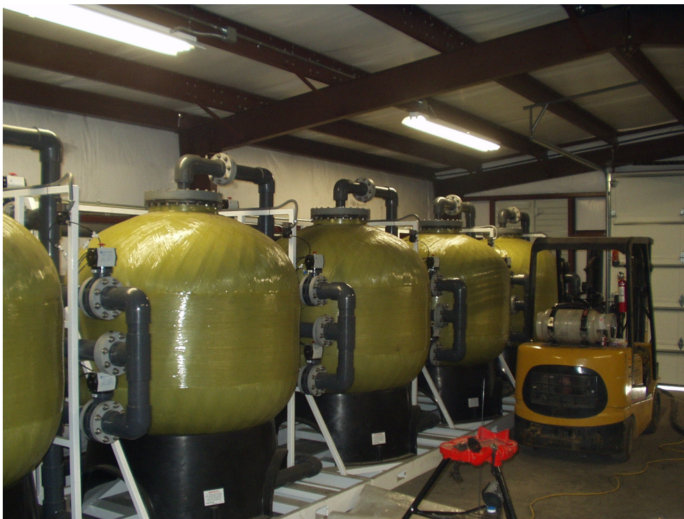
Picture 4: Filters that DMI-65 was installed in.
